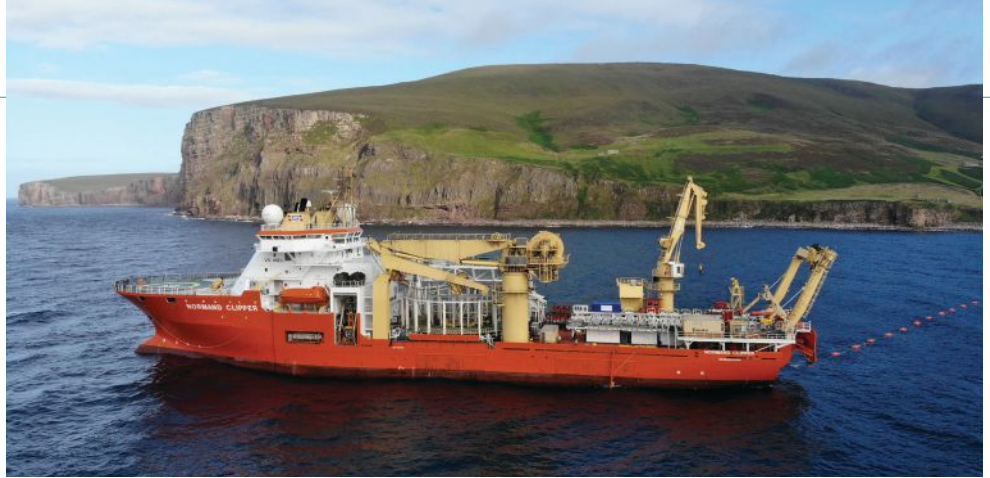
» A beach cable pull carried out by Global Offshore's Normand Clipper—a specialist cable installation vessel. (Photo credit: OceanIQ)
